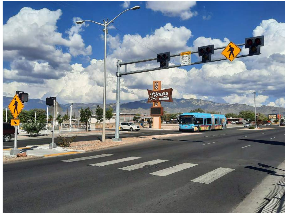
Recently installed PHB along Central Avenue near the International District Library
